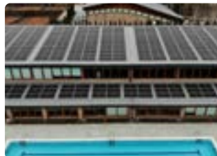
David Lloyd – solar PV installations
