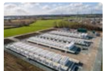
Pillswood – battery storage
