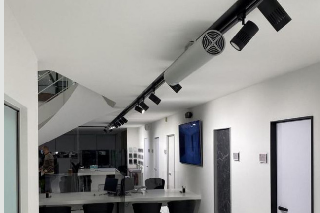
Installation of the Luxibel B Air V2 in the offices of Anyway Doors by Stage Unit
